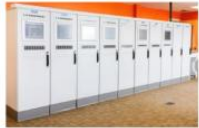
Instrumentation and Control
