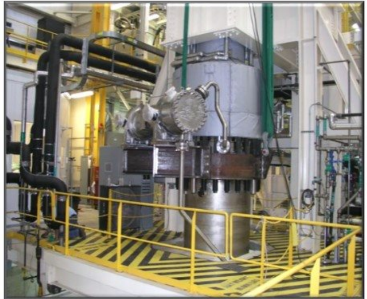
AP1000 RCP Test Facility
