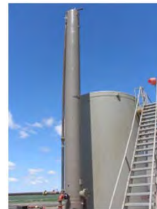
Vapor Recovery Towers
